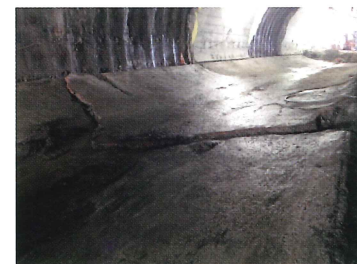
Photo 6 Differences in grade of invert concrete
