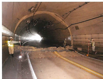
Photo 2 Compressive destruction and earth heaving
