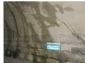
Photo 3 Openings and cracks caused by shearing force
