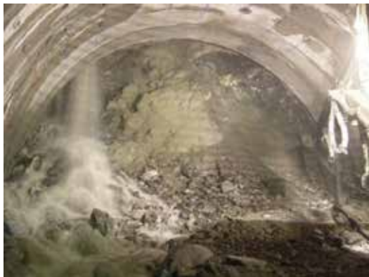
Photo 1 Water gush during tunnel excavation
