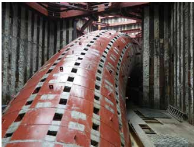
Photo 1 3D curved path of a discharge conduit
