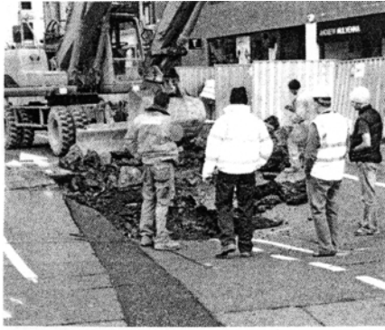
The damaged caused to the Road on Cromac Street in Belfast City Centre, after it collapsing into what is believed to be a large hole above a storm-water tunnel.
