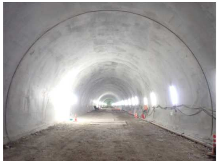
Picture-7 Surface Appearance (From inside)
