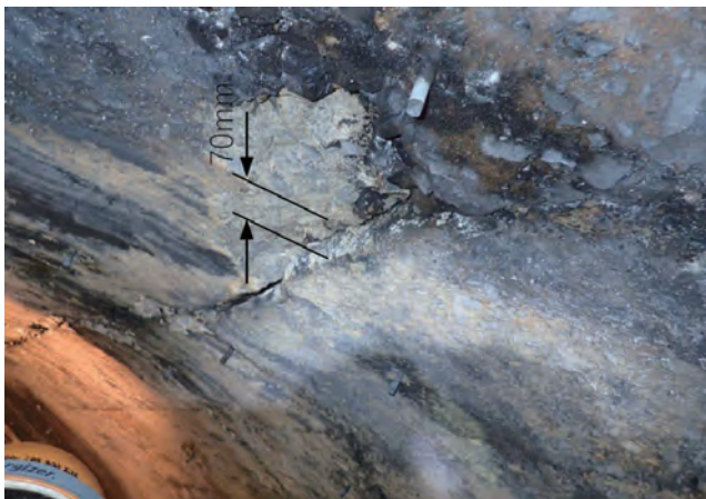
Photo 1 Portal deformed conditions
