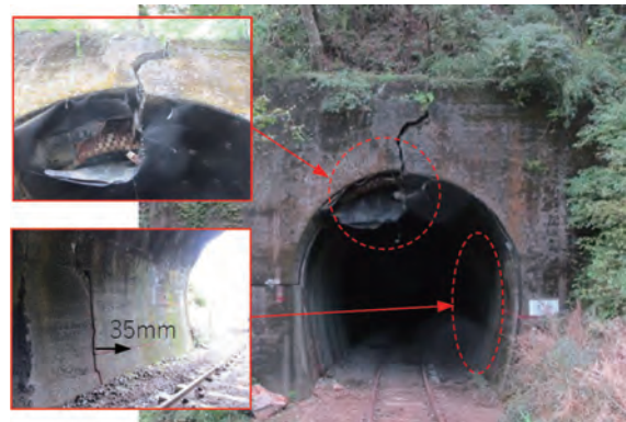
Photo 2 Lining deformed conditions
