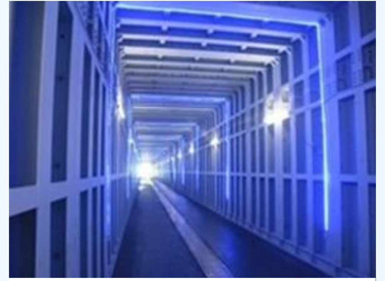
Photo 3 Lighting inside protector
