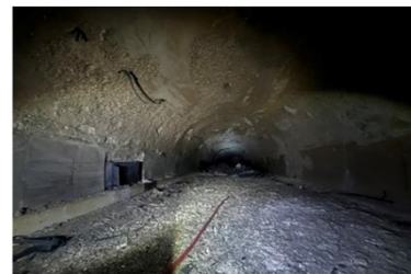
Photo-2 Amako-yama Tunnel Fire Damage
