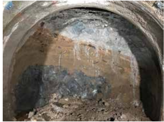
Photo-2.1 A Tunnel Face Sample in Japan with Soft and Hard Ground
