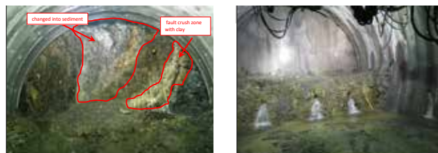
Fig. 2 Condition of the Fault Crush Zone during Excavation
