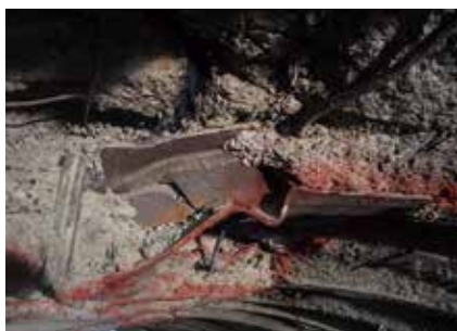
Photo 2 Buckling of steel support
