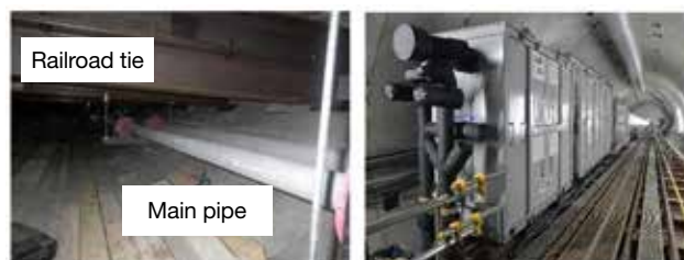
(a) Main pipe
