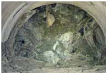
Fig. 1 Buckling of the arch supports
