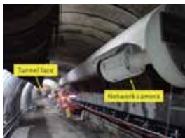
Fig. 2 Installed network camera
